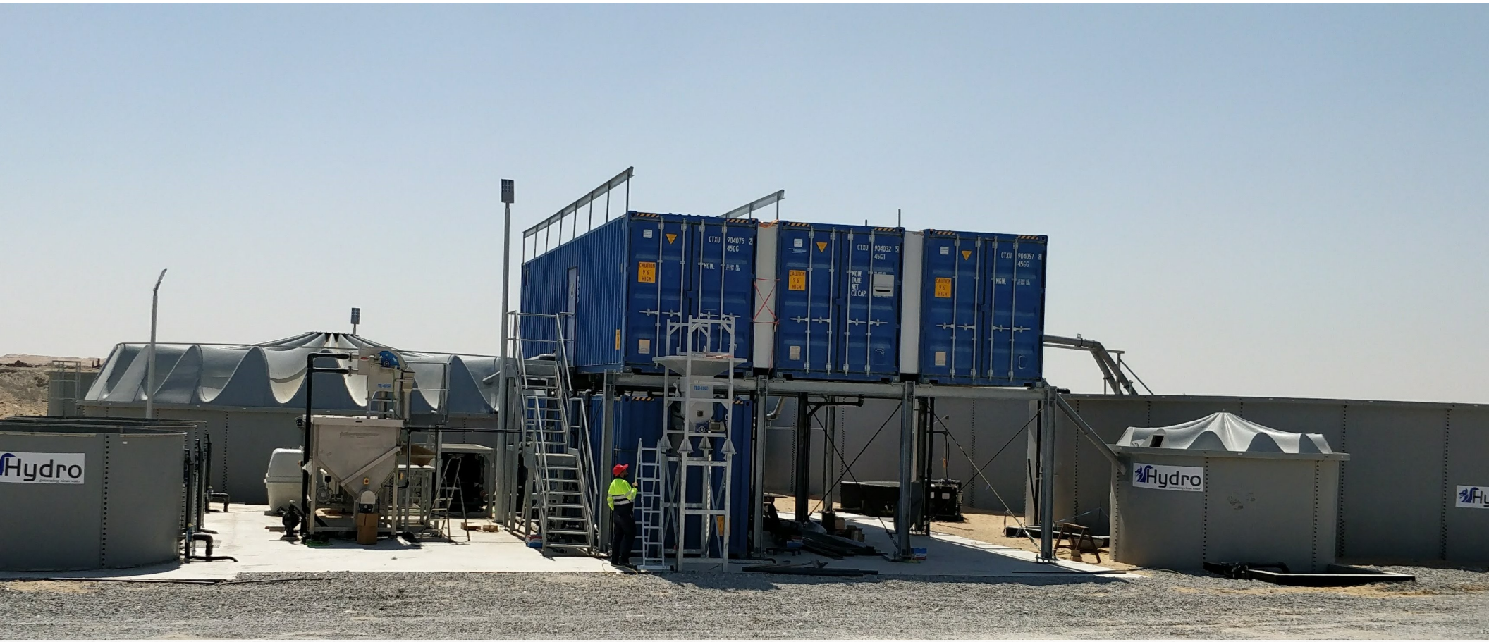
Industrial Waste Water Treatment Plant – 300m 3 / day
